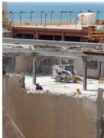
Phase 1 of San Onofre Nuclear Generating Station's demo took 16 months to complete.
